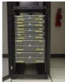
Dell "Rack" Servers
